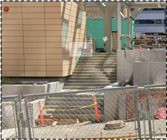
Existing stairs conflict
